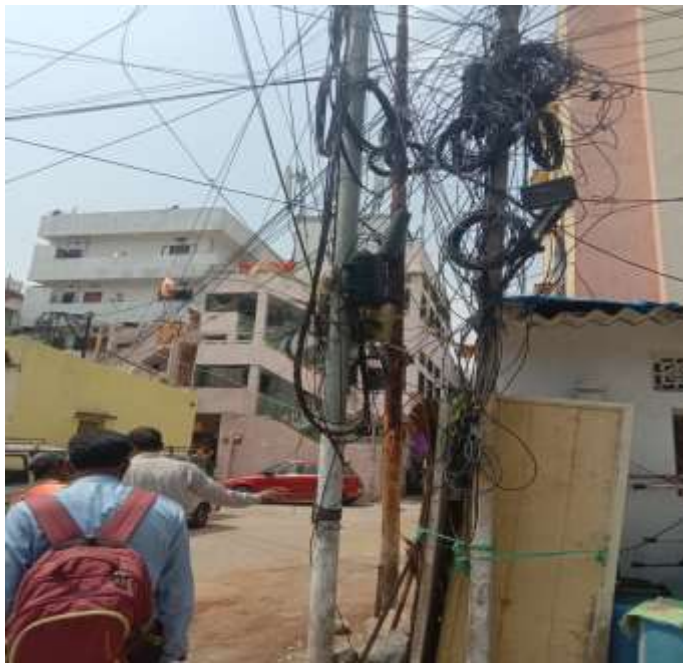
Figure 3: Clumsy electrical cables at Indira Nagar Colony.
