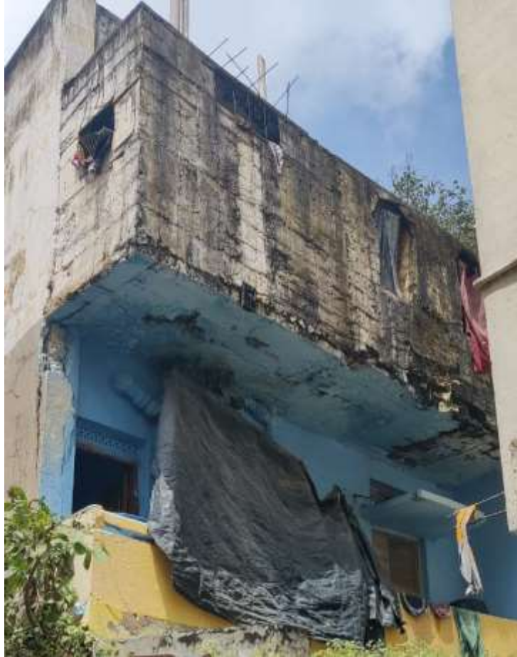
Figure 8: Cracked floors and chipped walls
