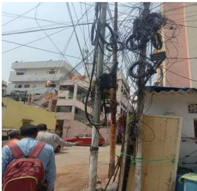
Figure 3: Clumsy electrical cables at Indira Nagar Colony.
