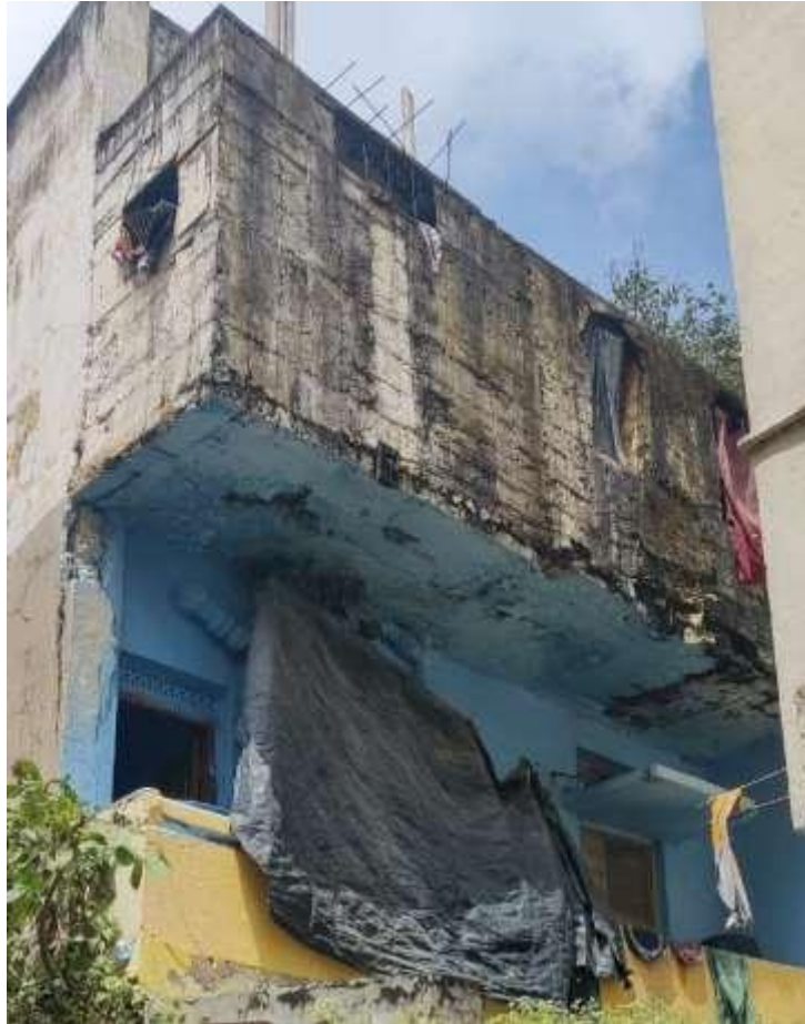
Figure 8: Cracked floors and chipped walls
